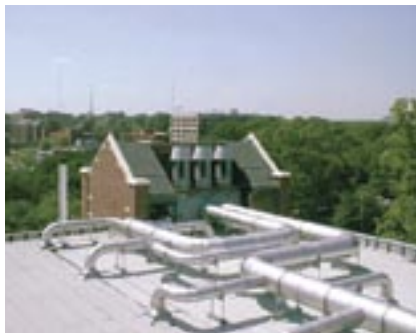
Photo 2: A mixed-flow impeller system on the roof of Georgia State University laboratories
