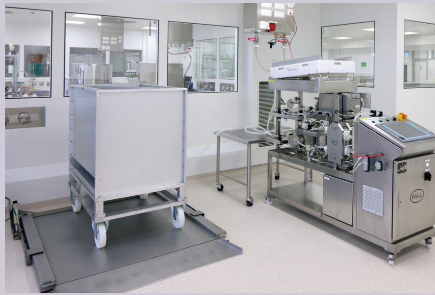
Photo 4: Manufacturing area for UF skid
