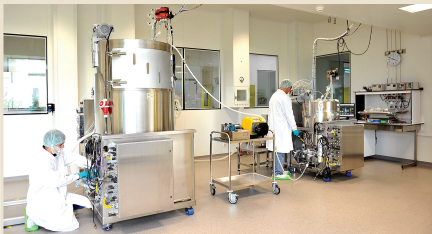
Photo 4: Upstream process area with a 25-L Wave bioreactor from GE Healthcare (RIGHT) and two Thermo Scientific HyClone SUB single-use bioreactors (250 L and 1,000 L); bioreactors are connected with utility panels from the ceiling. Media tanks are located outside in the material hall. The area was sized to include a second 1,000-L bioreactor.
