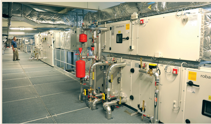
Photo 6: Technical plenum of the process areas; the conception was designed to ease maintenance. All HVAC systems are positioned just above their corresponding classified area to simplify duct work and increase efficiency.
