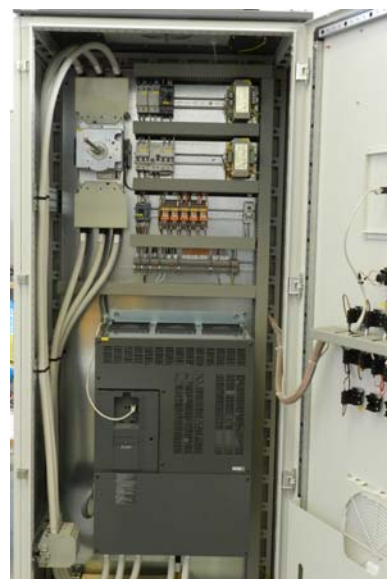
Inverter electrical cabinet example
