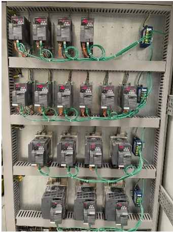
Image 4: The new door press application line was is run by 19 Mitsubishi Electric's FR-E series VSDs.
