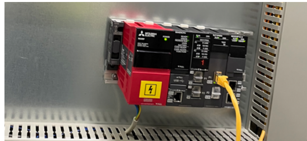
The Melsec I-QR series controller provides the operating data for the Asset Portal via the RD55 data logger. Source: Mitsubishi Electric Europe B.V.
