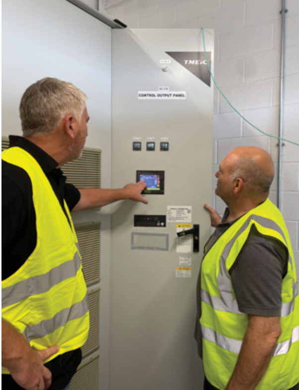
Operating data is visualized in a user-friendly way via the GOT operator terminal from Mitsubishi Electric. Source: Mitsubishi Electric Europe B.V.
