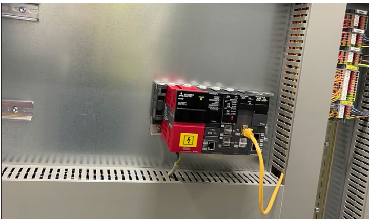
Image 7: The MELSEC I-QR series controller provides the operating data for the Asset Portal via the RD55 data logger.
