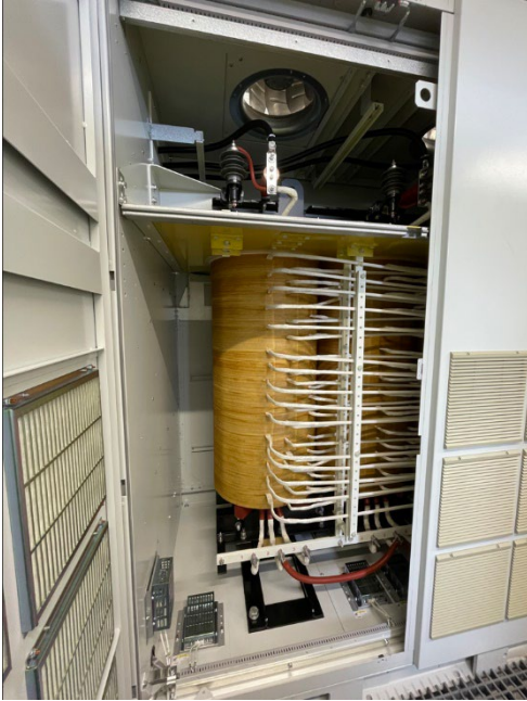
Image 6: The transformer ensures the power supply for the drive units.
