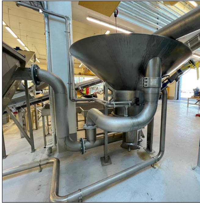
Figure 2. Sand washing machine in Veitur wastewater treatment plant in Klettagarðar.
