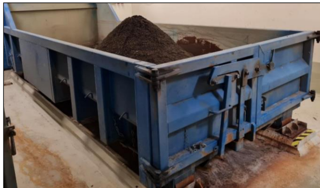
Figure 3. Cleaned sand in the waste collection area of Veitur wastewater treatment plant in Klettagarðar.
