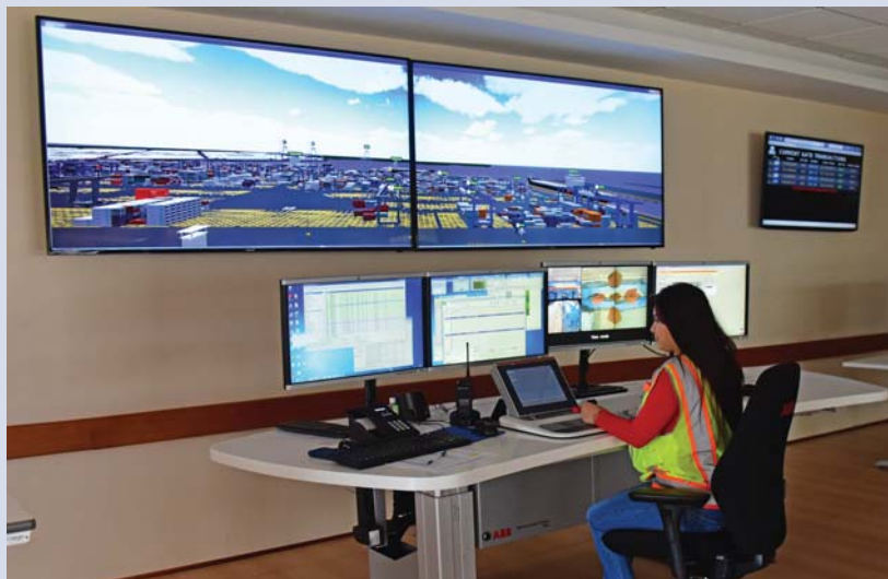
Control room for automatic cranes
