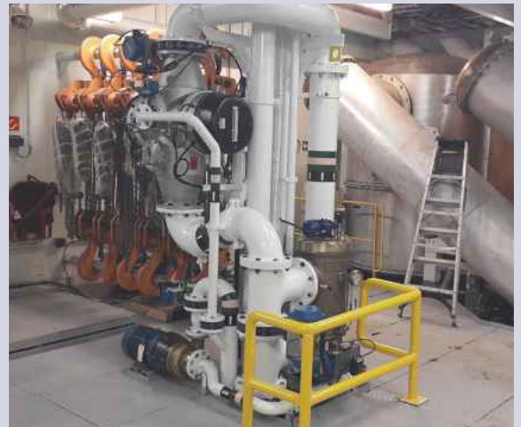
Hyde Marine Guardian-US system in-situ
