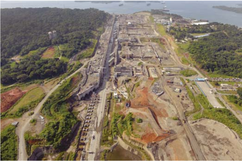
Construction of the new Agua Clara locks in the Atlantic side (September 1, 2014)
